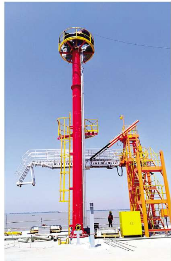
Foam Monitor Tower, PSW Terminal Project
