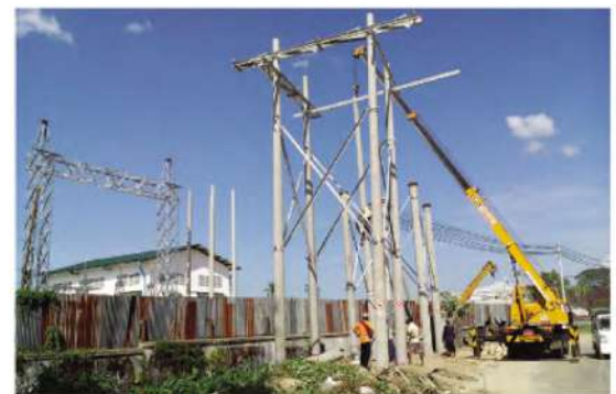
11 kV Distribution Line
