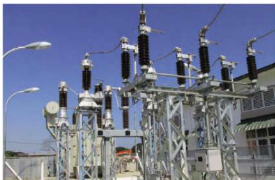
66/11 kV, 10 MVA Substation
