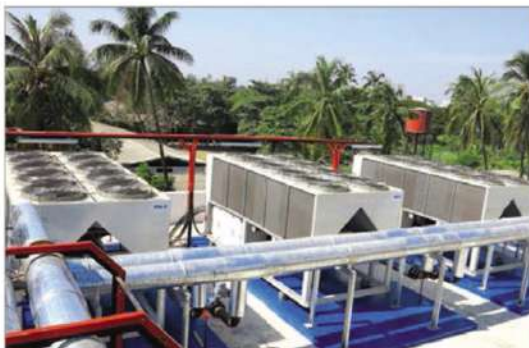
Air Cooled Chiller
