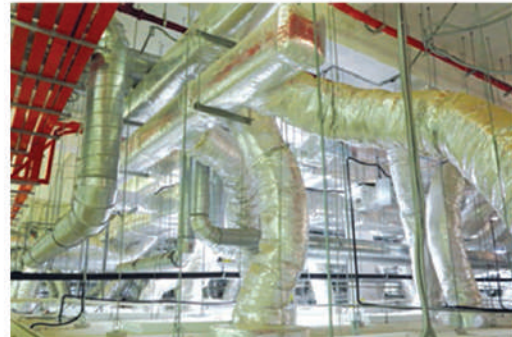
Ducting and Piping
