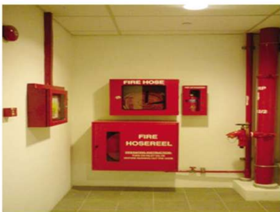
Fire Fighting Equipment
