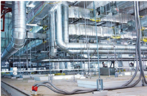
Ducting and Piping
