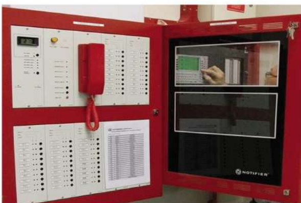
Fire Alarm and Intercom
