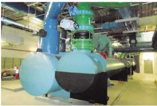
Water Cooled Chiller
