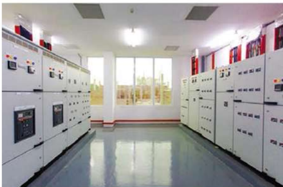
Electrical Main Distribution Boards
