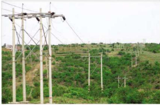
66 kV Transmission Line (MyinGyan-Nabuai)
