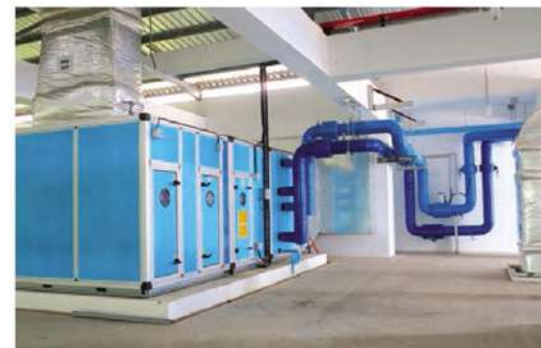
Air Handling Unit
