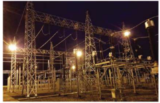
225 MW Combine Cycle Power Plant Project
