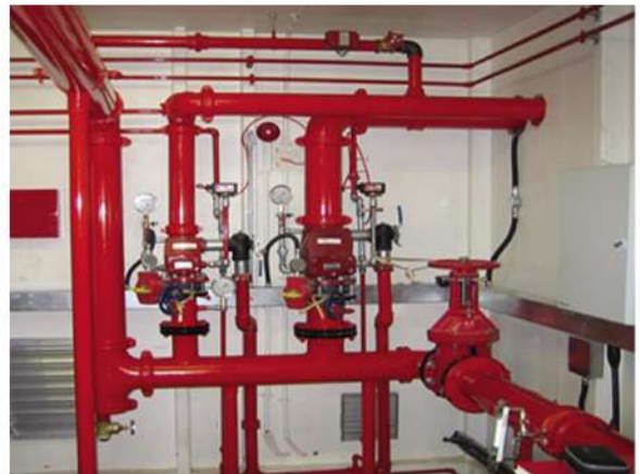
Sprinkler Control Valves
